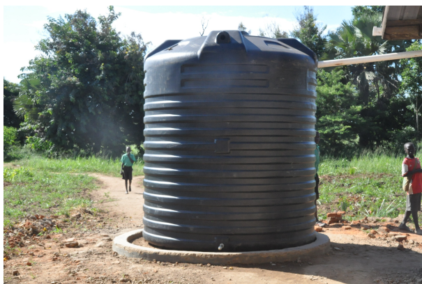
The 10,000 water tank at Abone primary school.
